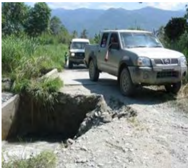
Picture 24: Washout on the Kokoda National Highway
