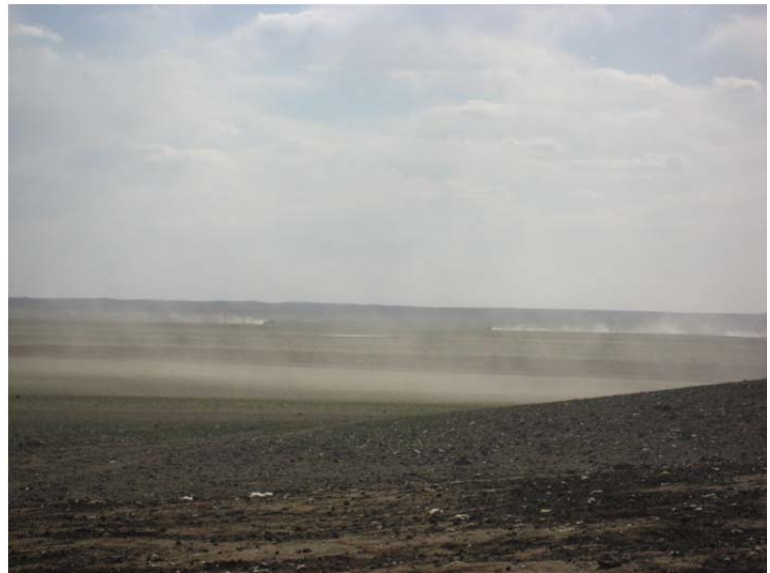
Figure 14. View from Ger impacted by construction of water pipeline.
